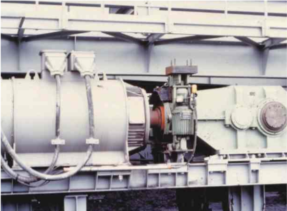
GEAR / FACHINI (Milano - Italy) Gearbox - Cement Plant
